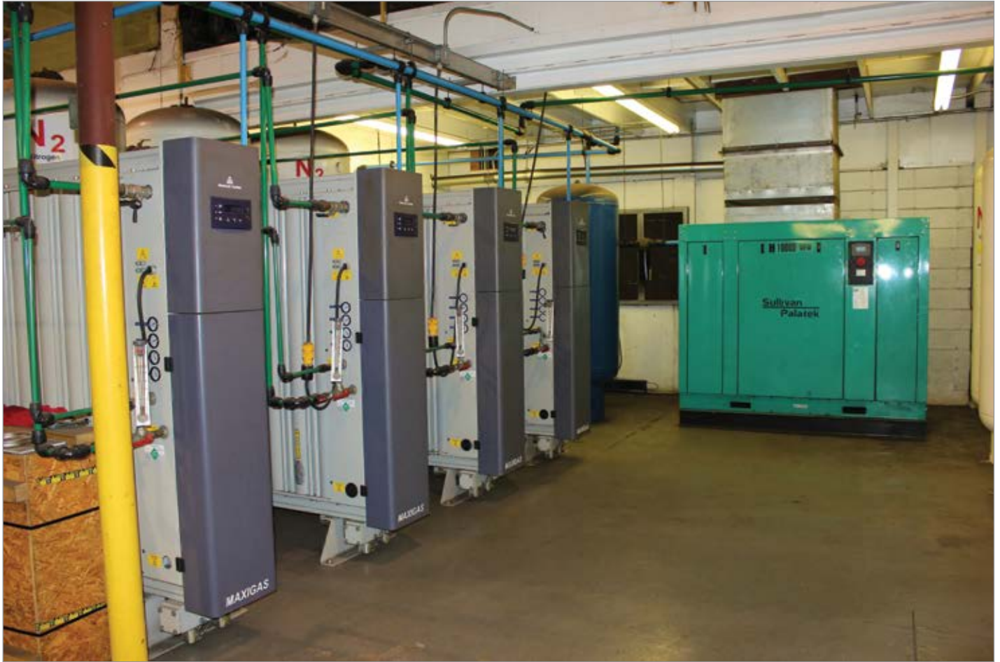
A complete on-site nitrogen generation system.
