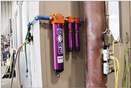
Tsunami CORE Series Desiccant Dryer installation.
