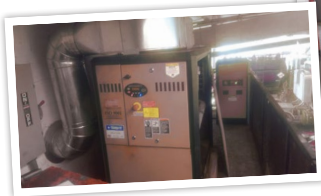
No doubt floor space was tight for this Seattle metro manufacturer, but plan for easy access when installing a compressed air system.
