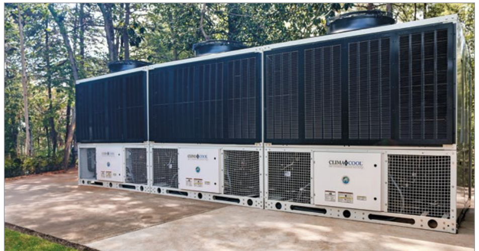
Three 20-ton air-cooled simultaneous heating and cooling modules conditioning an office building. No boilers or cooling towers were needed.
