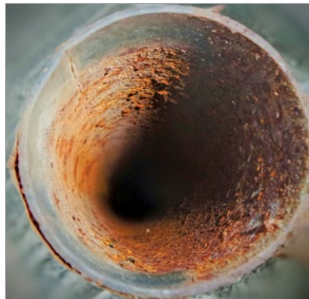
Humidity can cause damages in a compressed air system, e.g. rust.
