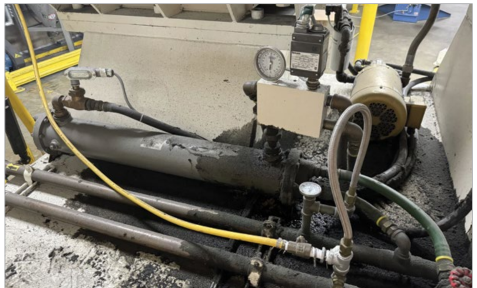
Gearbox oil cooler equipped with thermostatic control valve (in box with gauge) and leaving oil temperature sensor in fitting at other end of heat exchanger.
