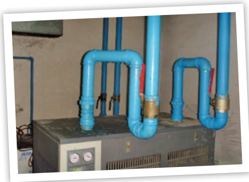
The U-turns in the steel piping leading to this refrigerated compressed air dryer cause pressure drop.
