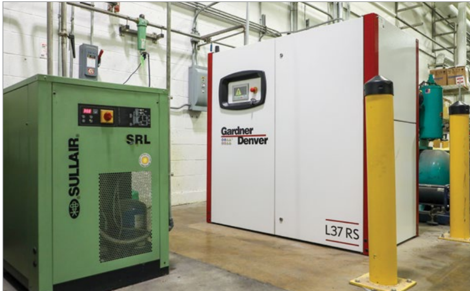
Tröegs's rotary screw air compressor installation
