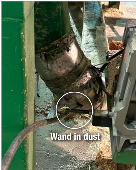
Figure 5: A blow wand stuck in a sawdust recovery duct blows constantly, even during production downtime. This application could be eliminated with proper ducting.
