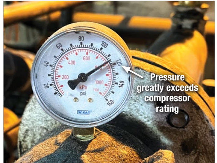
Figure 1: The pipes connecting this 200-hp air compressor to the remote cooler installed on the air compressor room wall were only two-inch size, causing a large pressure loss. Because the air compressor is only rated at 100 psi (7 bar), the drive motor would trip.
