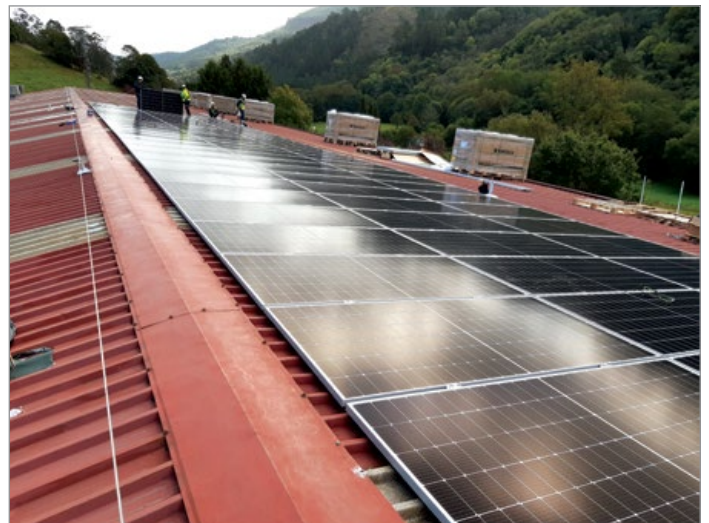
One of Klöckner Pentaplast's energy efficiency projects was installing solar panels at its facility in Asturias, Spain.
