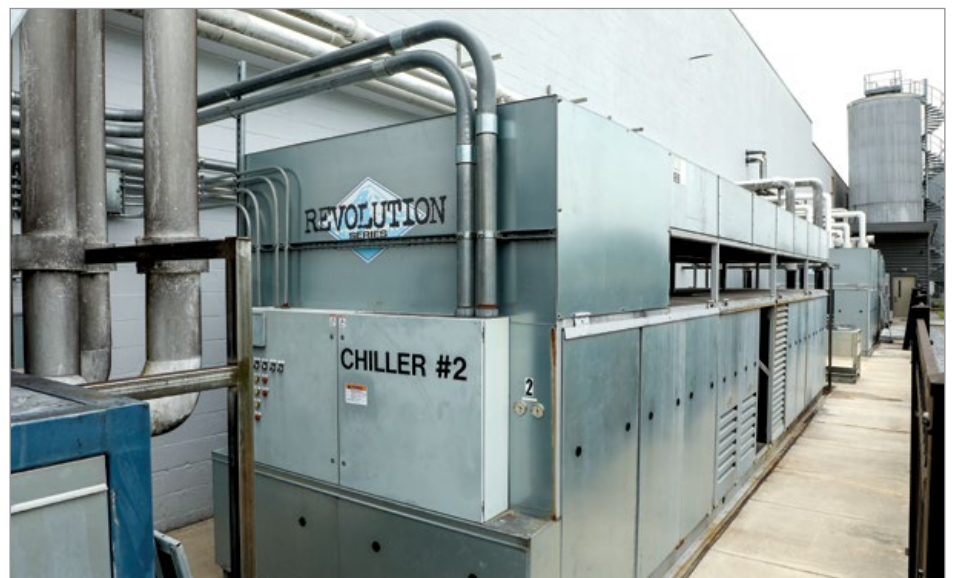
Tröegs's three chillers from Pro Refrigeration keep the beer and yeast at a stable temperature for production.
