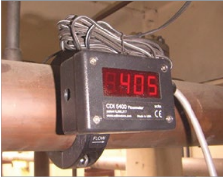
A thermal dispersion flowmeter installed on piping in a plant.
