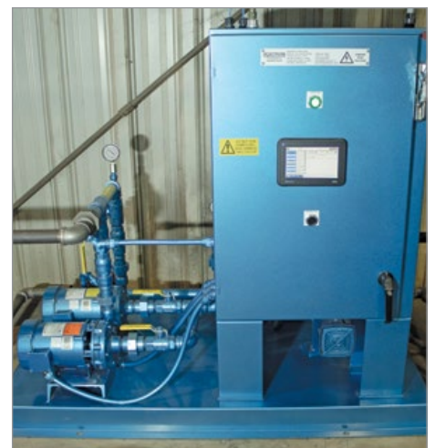
The advanced control panel mounted to a pump and control skid
