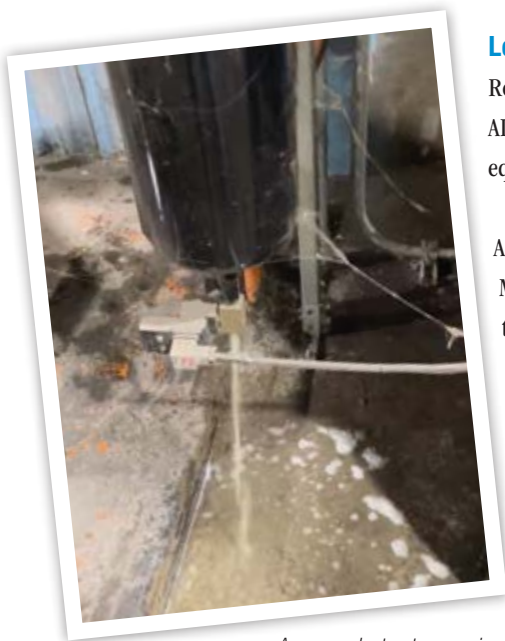
A power plant got a surprise when testing this desiccant compressed air dryer, thanks to a leaky bypass valve.
