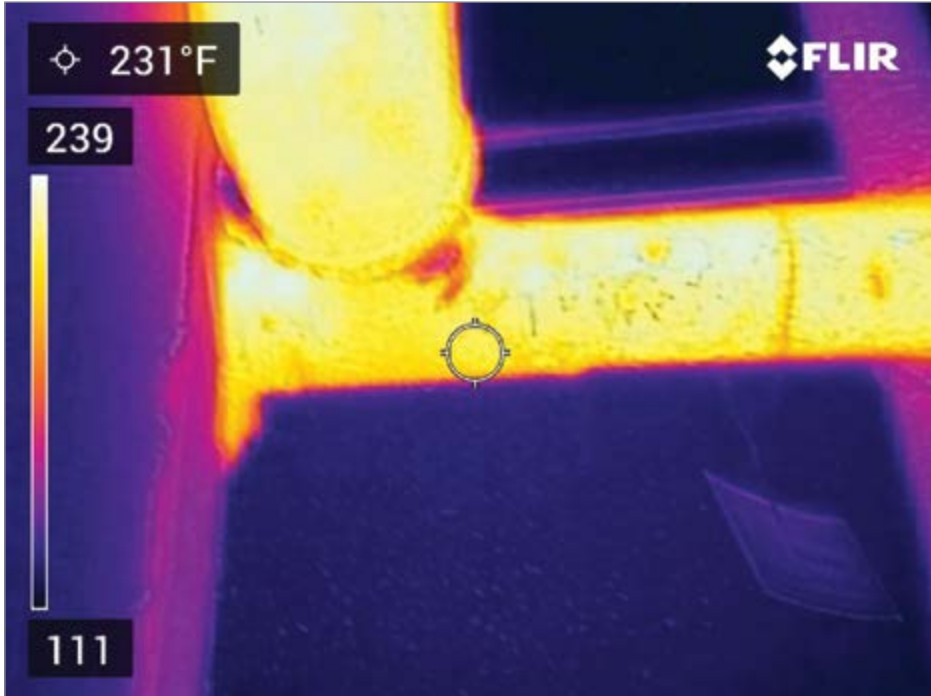
Neglecting insulation repairs, such as on this uninsulated steam line, can cost more than it saves.
