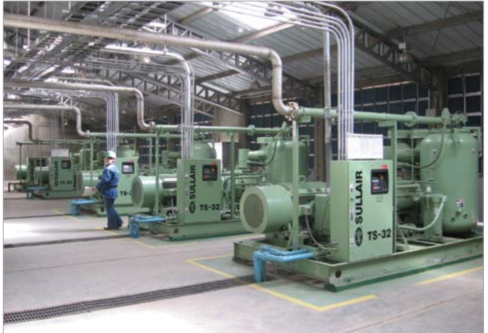
Secada preferred installing air compressors without cabinets, as it made maintenance easier.
