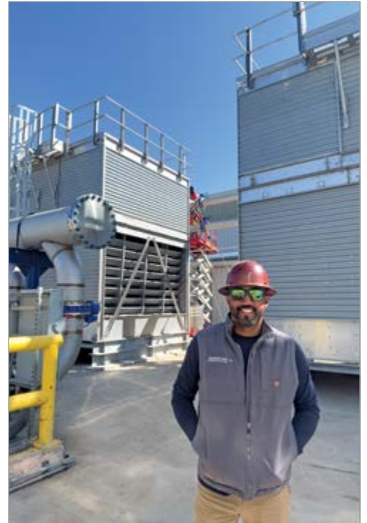
ETS Project Manager David Ramirez with the installed cooling towers
