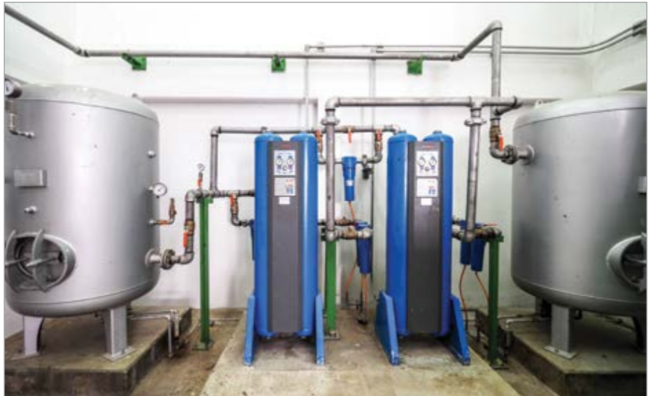
Demonstrate how putting off repairs – such as fixing compressed air leaks – hurts financial performance.
