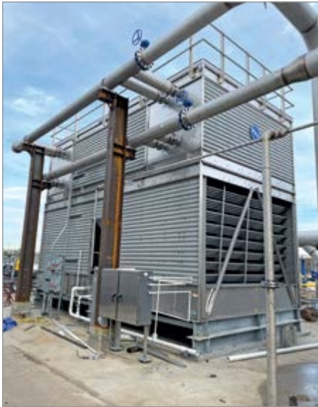
A BAC FXV combined flow cooling tower anchors the closed loop cooling system.
