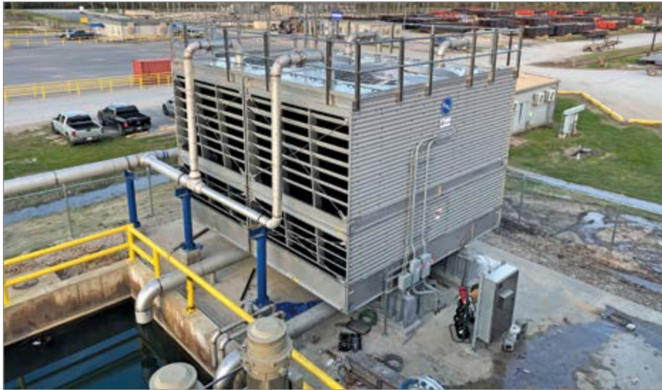
The open loop system's crossflow cooling tower
