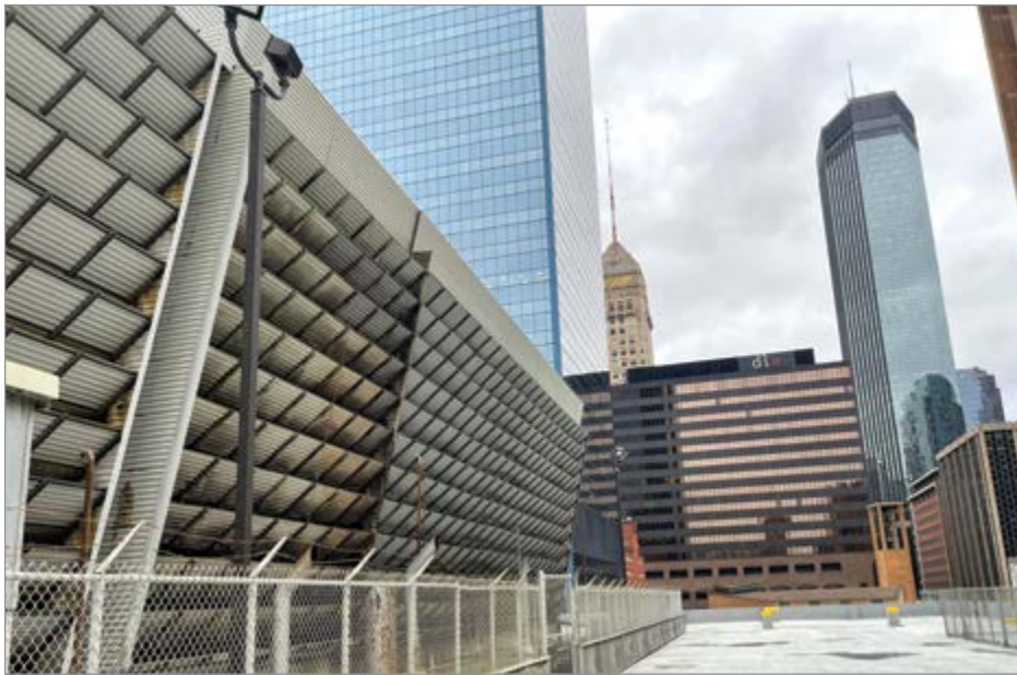
A view of the rooftop crossflow cooling towers. Most of the buildings shown, including the IDS Center at right, are district energy system customers.
