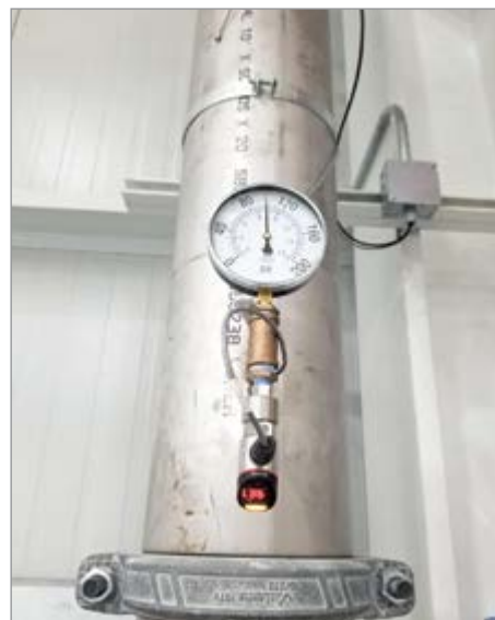
A compressed air system's main header pressure gauge
