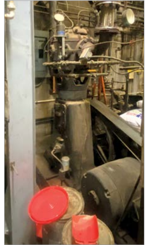
The plant's compressed air system included this older reciprocating air compressor.
