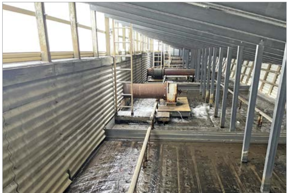
Inside the main plant’s crossflow cooling towers.
