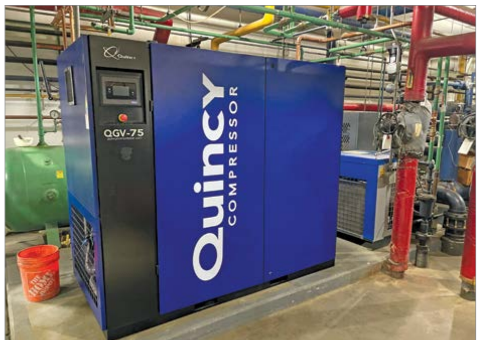
The main plant uses air compressors to start its CAT engines and run pneumatic controls.
