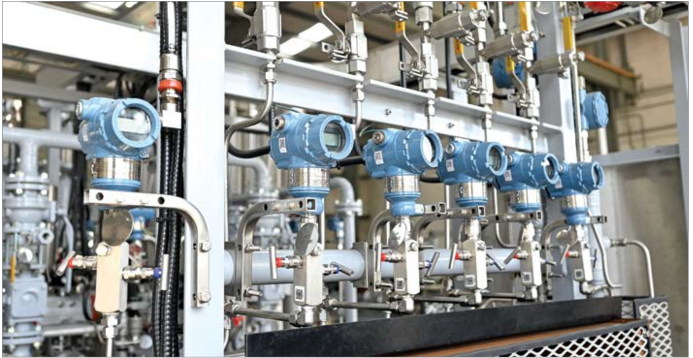
A nitrogen generation system customized to meet customer-specified instrumentation and tubing requirements.
