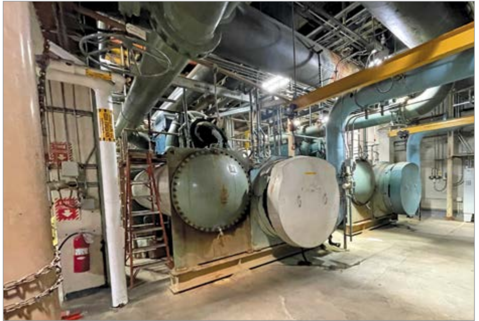
Shell-and-tube centrifugal chillers in the district energy system’s main plant.
