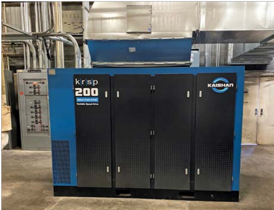
A 200 horsepower VSD rotary screw air compressor
