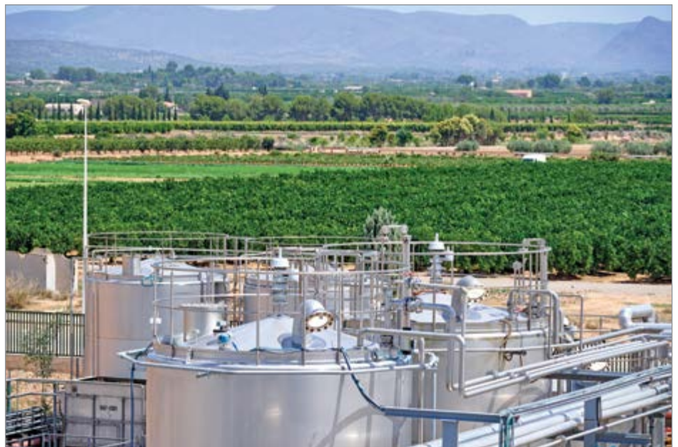
Kensing’s Valencia facility (Photo: Jaime Brotons)
