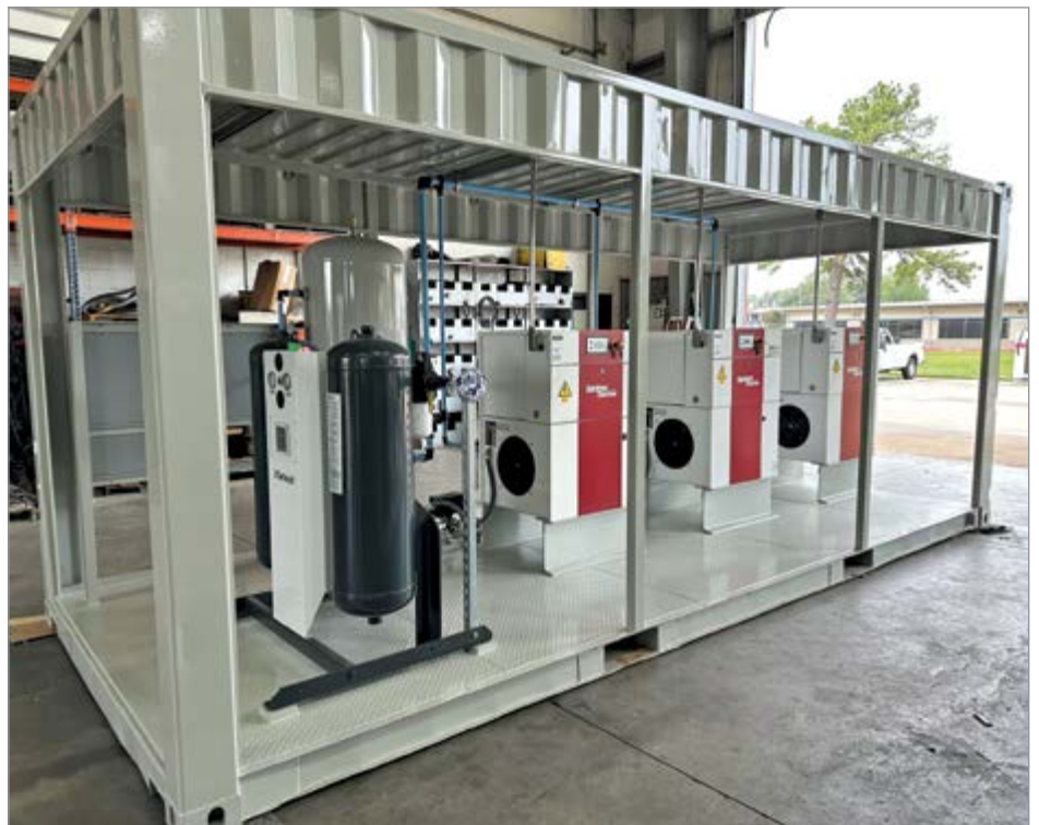
Three air compressors and a heatless desiccant air dryer in one container wired for a single power feed.
