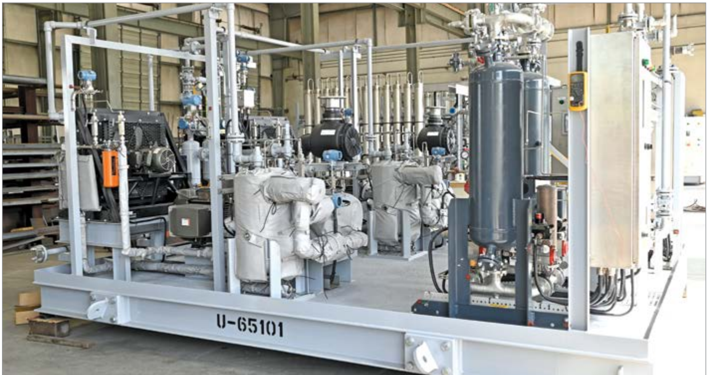
This skid contains two 60 HP air compressors with two heatless desiccant compressed air dryers.
