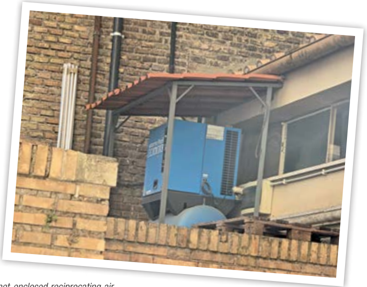
This cabinet-enclosed reciprocating air compressor powers a woodworking shop in the Vatican City.
