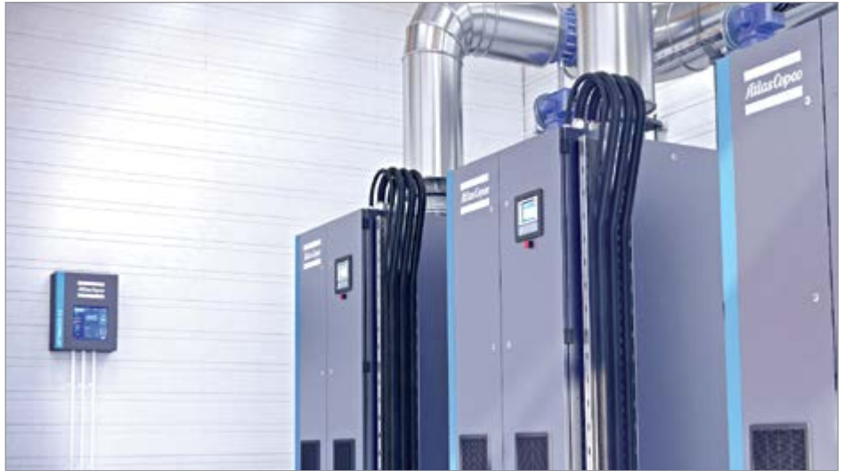
This compressed air system controller is integrated in an air compressor room for centralized compressed air system management. Energy consumption can account for up to 70-80% of an air compressor's lifetime costs.
