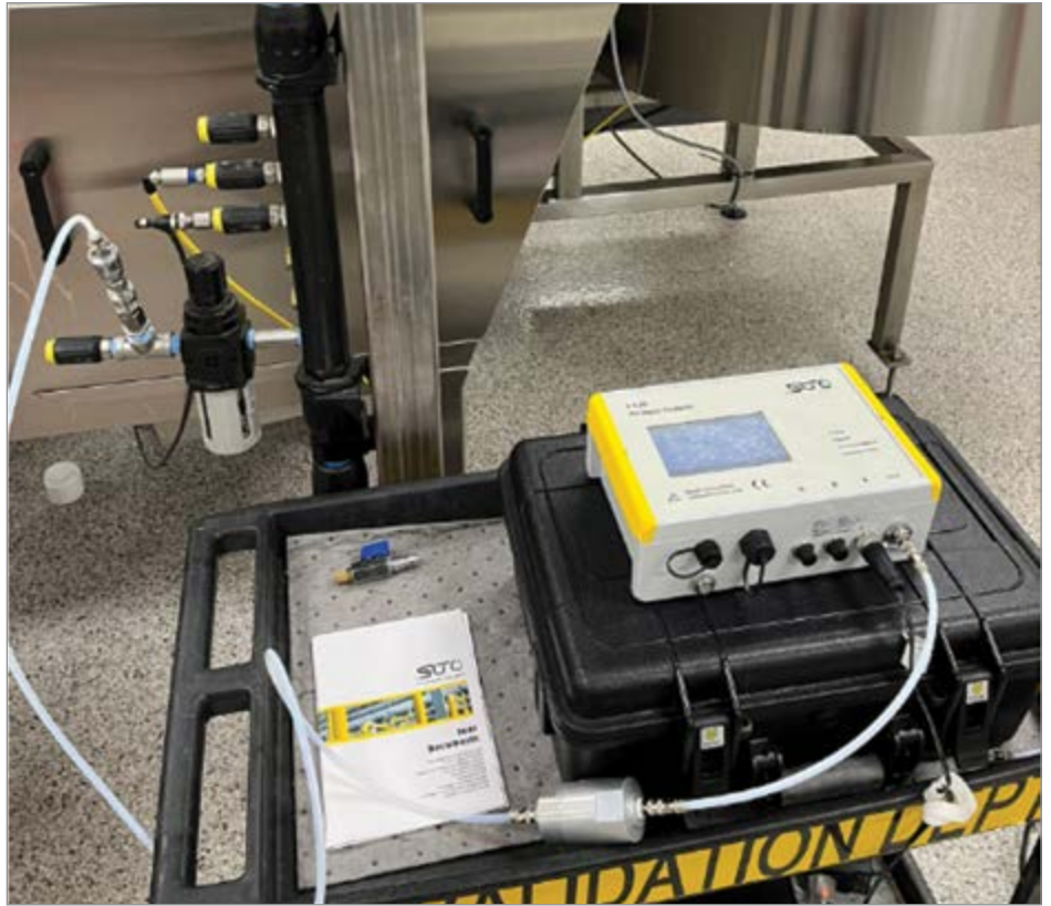
A measurement device ensured the compressed system met ISO 8573-1 Class 4.4.4. (Source: SUTO iTEC)
