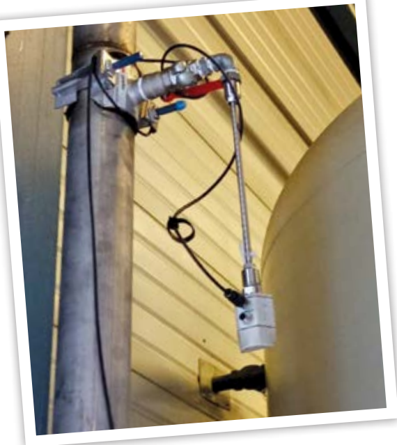
Using sensors to monitor compressed air system flow only works if the sensors are installed correctly.
