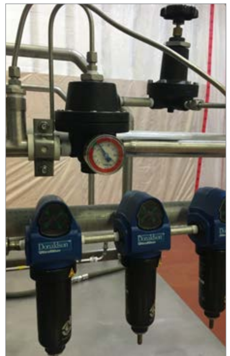
Secondary filters were required due to contamination from lubricated air compressors.
