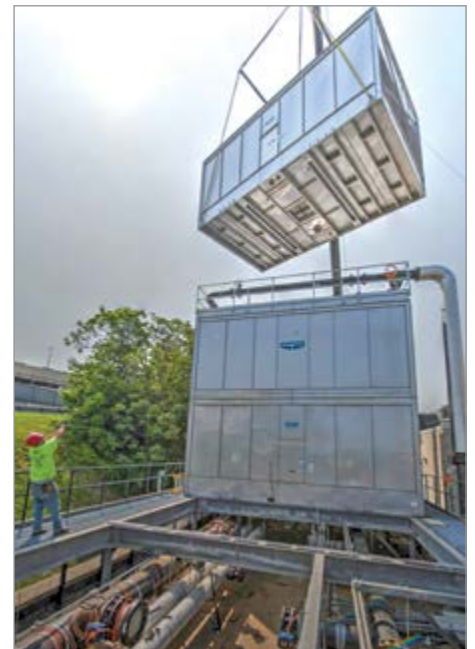
A crossflow cooling tower rigged and assembled on-site, highlighting the precision and teamwork required for proper installation.
