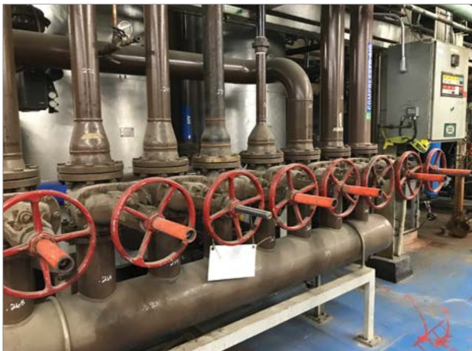
Compressed air average pressure, flow and dew point is measured and monitored.
