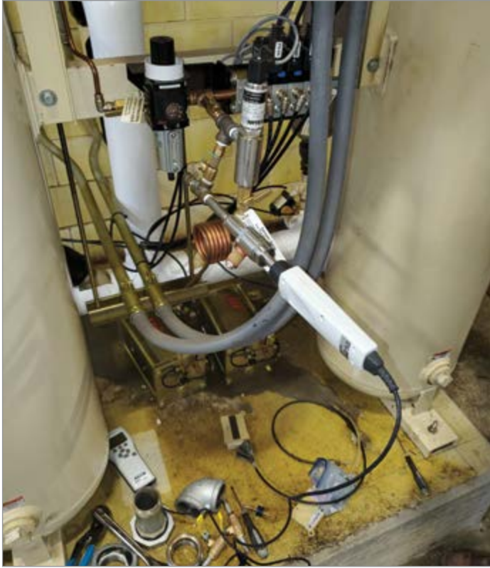
A second calibrated dew point monitor verified the accuracy of the PDP reading and showed the oil had damaged the dryer's dew point monitor.
