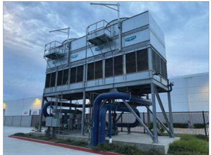
A 1,380-ton EVAPCO open cooling tower supplies cooling water to two water-cooled Trane centrifugal chillers, which further cool tower water for delivery to process machines at rPlanet Earth. The tower also supplies cooling water directly to the facility’s compressed air system and equipment that doesn’t need chilled water at a lower temperature than that provided by the chillers.
