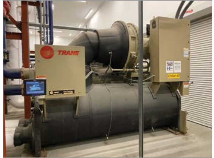
Trane’s centrifugal chillers at rPlanet Earth’s plant use an enhanced-flow management package, which allows them to deliver chilled water at targeted temperatures at an increase in flow of up to 50% per minute.
