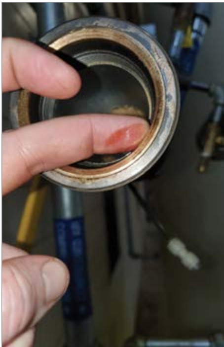
Oil in the compressed air piping downstream of the dryer pointed to the potential problem with the desiccant dryer’s inability to maintain the proper PDP.
