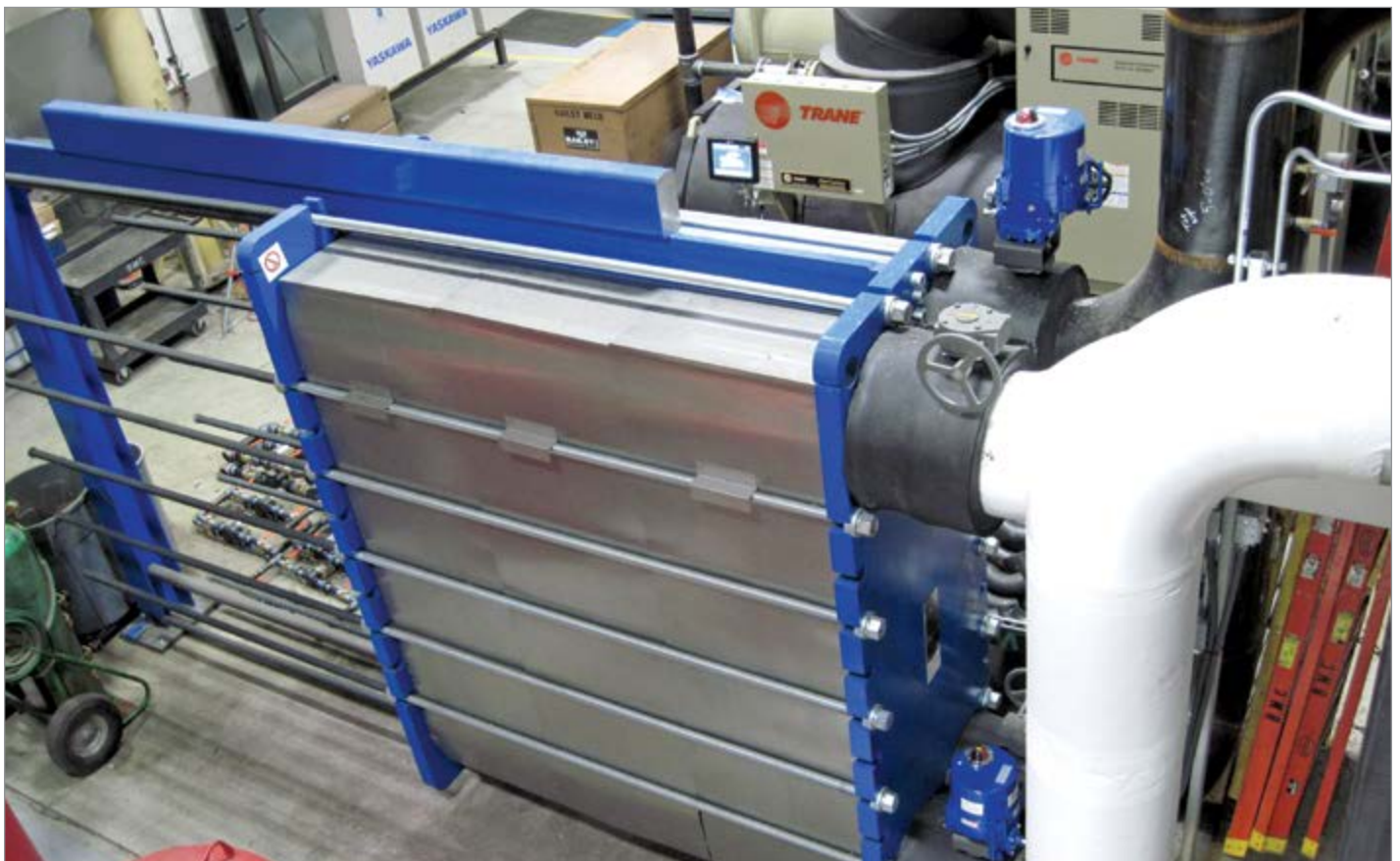
A 1600 ton free cooling heat exchanger with separate modulating control valves on cooling tower water and chilled water connections
