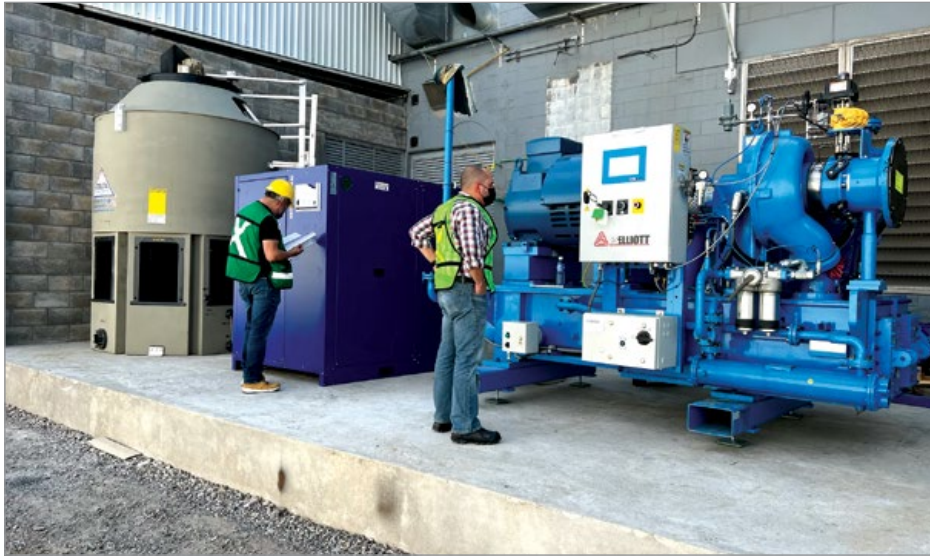
Daniel Mejia examines the installation of an 800-hp FS-Elliott centrifugal compressor in a textile company in Mexico.
