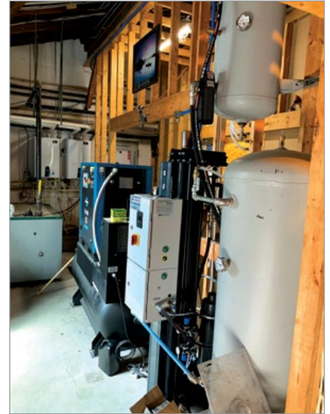
Mikropor MNG-US-35 nitrogen generator fed by a Kaishan KR5B air compressor
