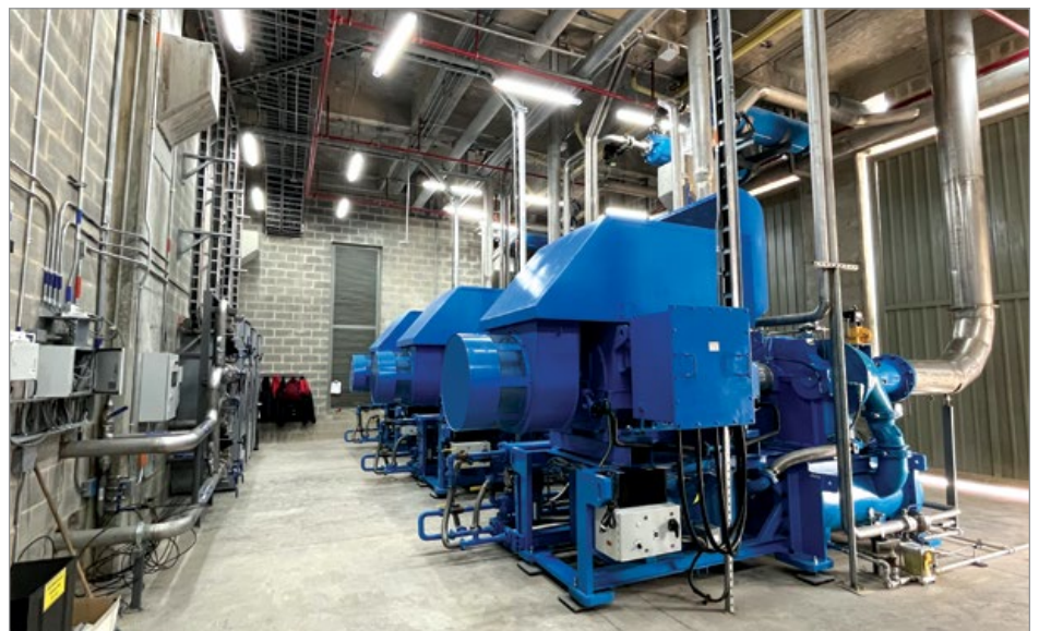
Three centrifugal compressors at a glass manufacturer
